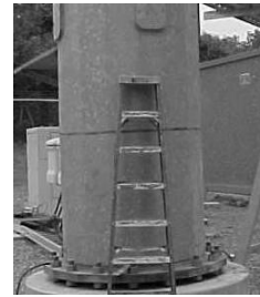
Improper Ladder use
