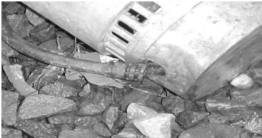
Defective Wiring on Capstan Hoist
